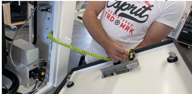
Figure 12 Connection of the grounding to the Right Panel.
