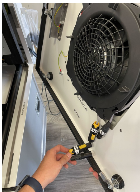
Figure 26: Connection of FAN A.
